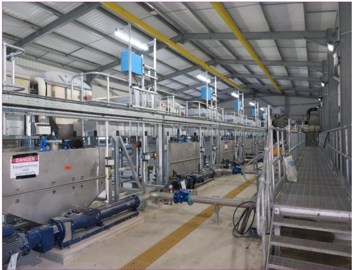
Figure 2-11: Thickening Building Knostrop sludge treatment centre
