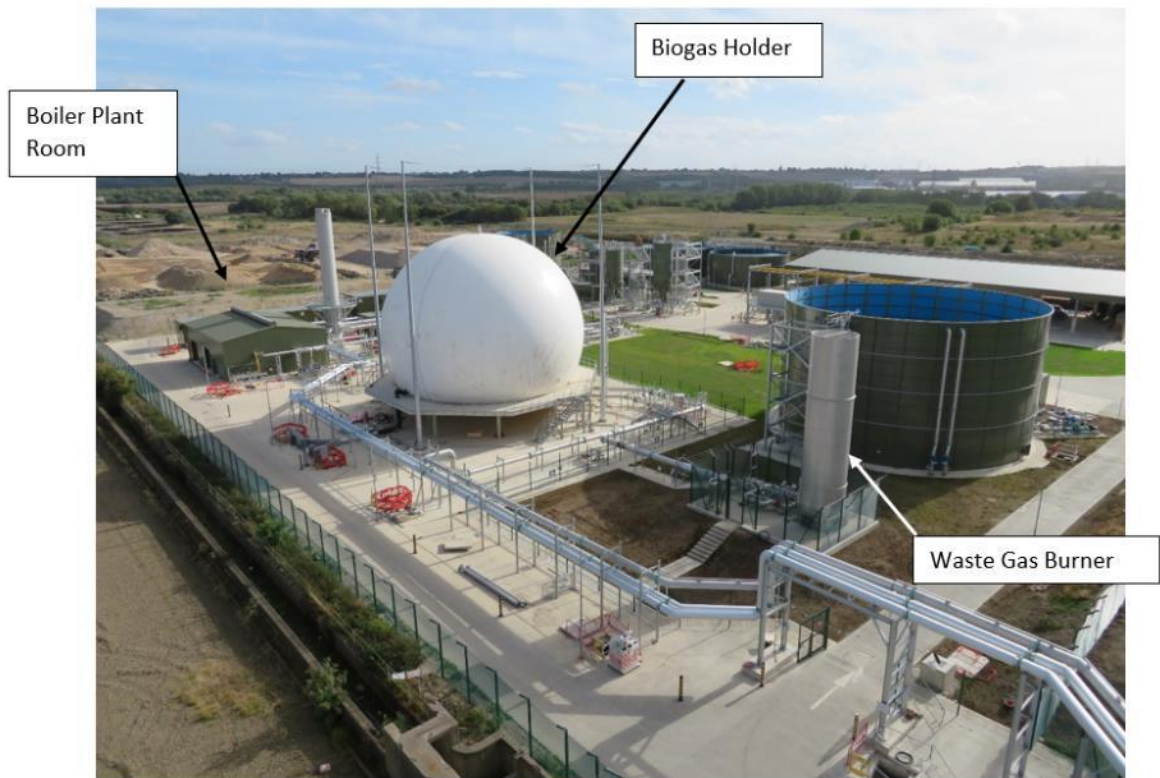
Figure 2-16: Knostrop sludge treatment centre
