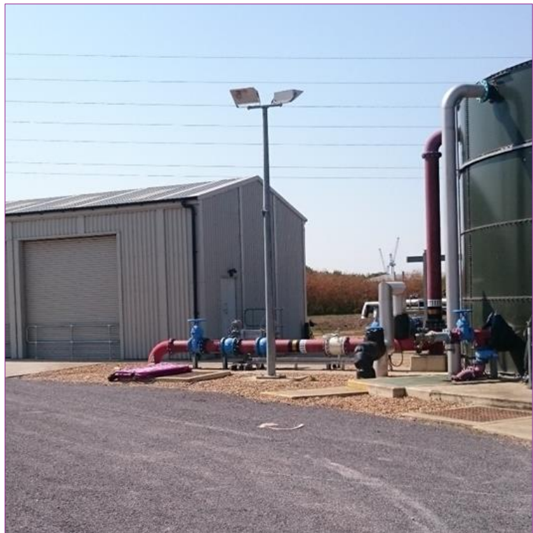
Figure 2-20: Example lighting unit
