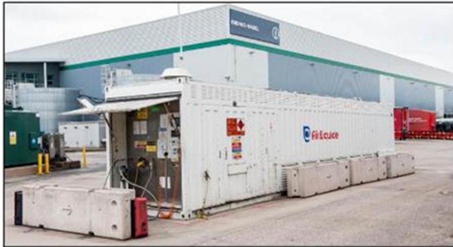
Figure 2-17: Typical containerised LNG facility
