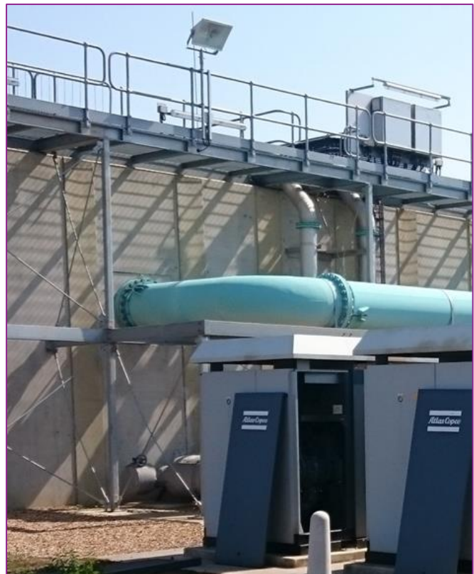
Figure 2-19: Example task lighting
