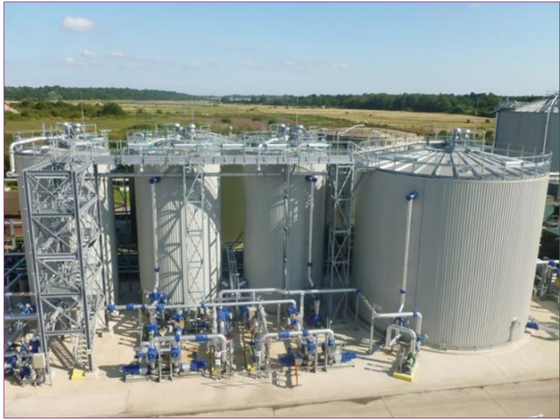
Figure 2-13: Colchester heating, pasteurisation and hydrolysis (HpH) process tanks
