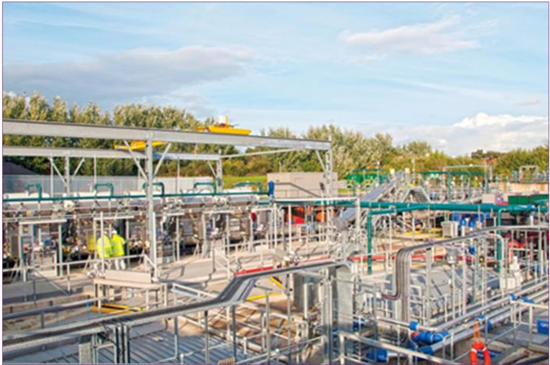
Figure 2-6: Mogden WWTP (West London) inlet works
