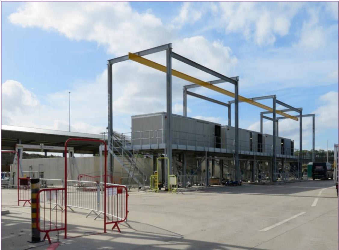
Figure 2-15: Sludge Dewatering at Knostrop sludge treatment centre
