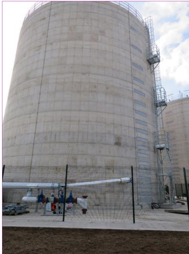
Figure 2-14: Digestion Tank at Knostrop sludge treatment centre
