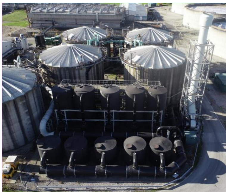
Figure 2-12: Hull STC Odour Control Plant
